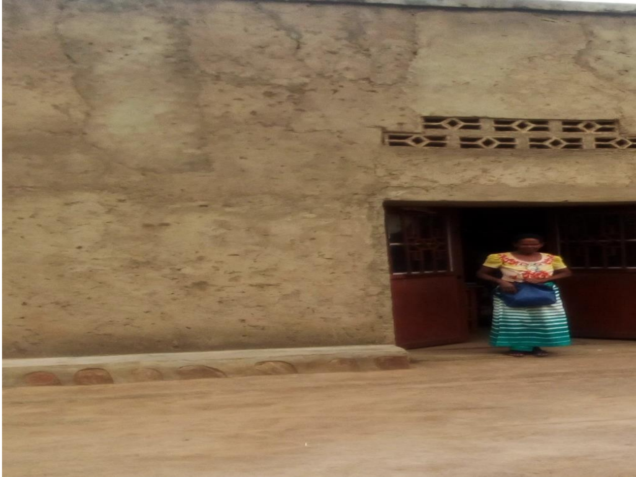
Figure 17: Dilapidated storage facility owned by CODEMATA
