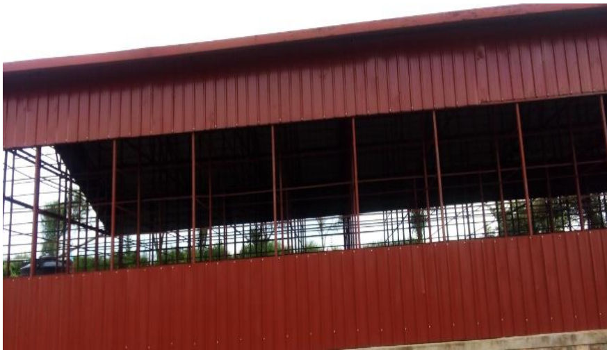
Figure 15: PASP-assisted modern drying facility in Kagiragi village owned by Ejoheza Cooperative
