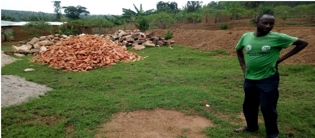
Figure 2.8: President of Koairu Ganza Cooperative standing close to the site where PASP has earmarked for the construction of the Cooperative’s storehouse. The bricks, gravel and tipped sand lying to his right.
